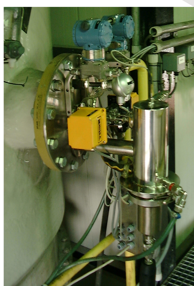
Figure 3: sampling unit installed at the hazardous waste incinerator
